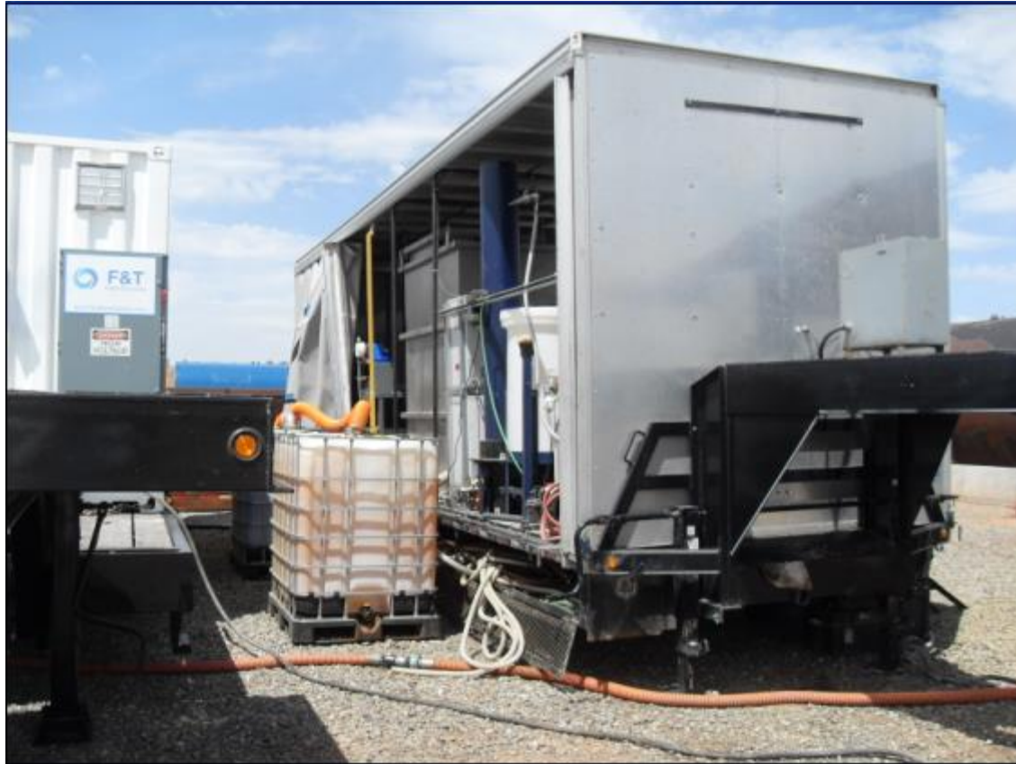
DAF equipment side view – pumping from 275 gal storage tank
